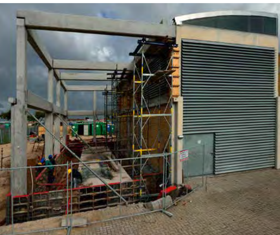
The upgrade of the Gugulethu substation was one of the key projects in the year under review.
