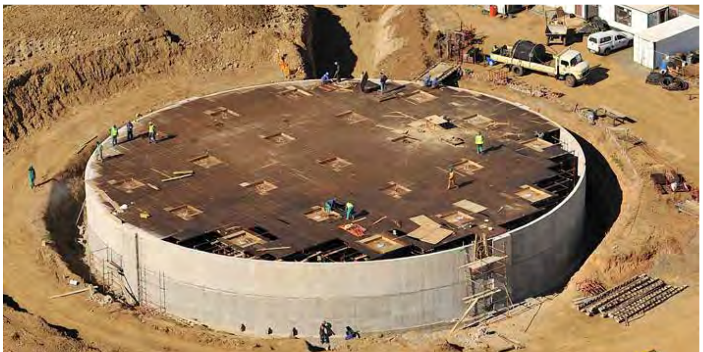
Once completed the De Grendel reservoir will provide 48 hours' worth of potable water storage capacity.
