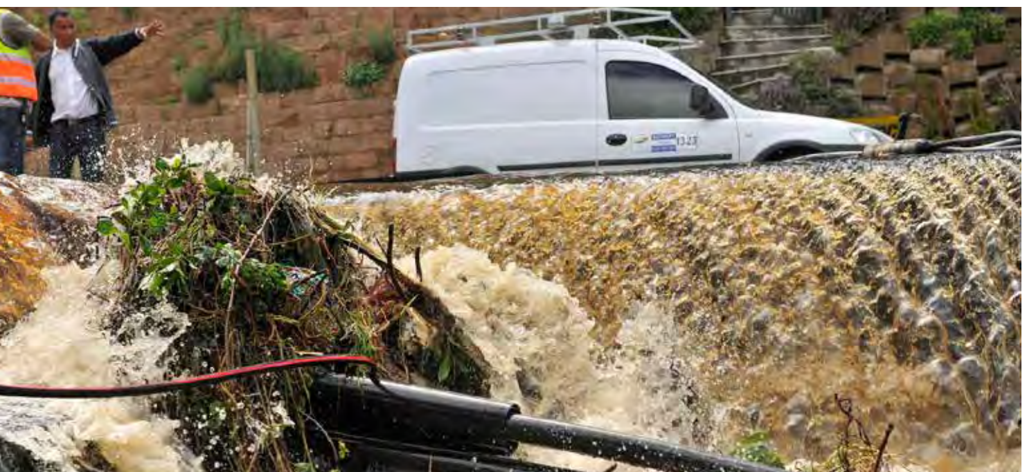
The City's stormwater infrastructure network requires large capital input to deal with historical inadequacies and damage caused by floods.
